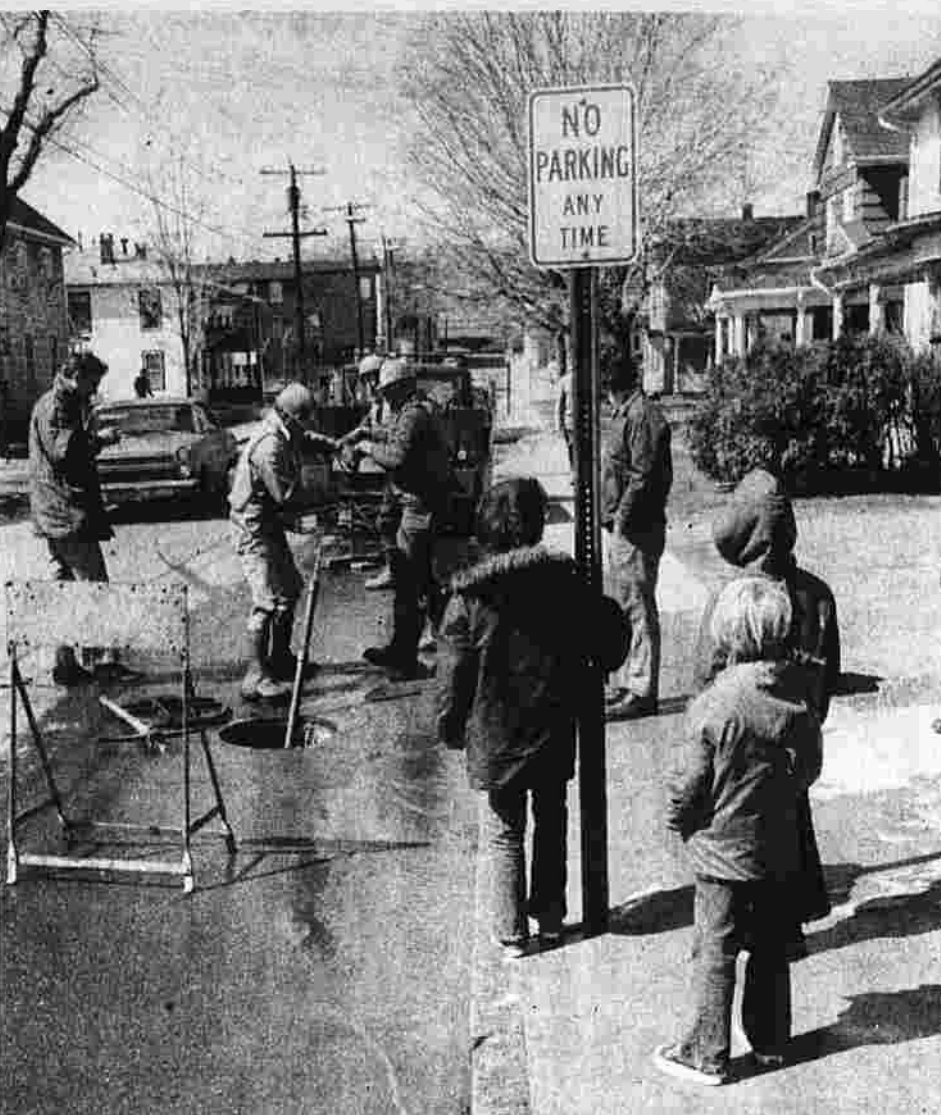
The crew from the town sewer department runs a metal snake into a sewer drain pipe under Birch St. at noon Friday. The snake worked. Within minutes of the crew's arrival, sewage flowed freely where it belonged, in the pipe.
